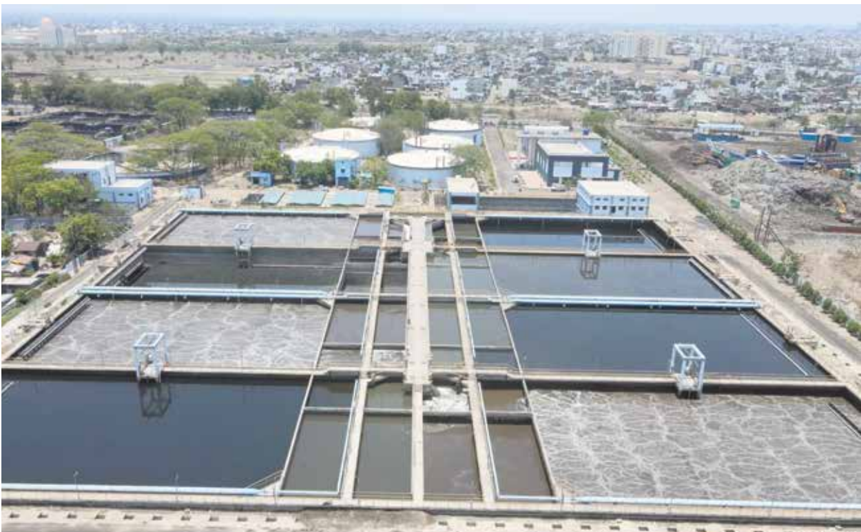
Koradi Sewage Water Treatment Plant
