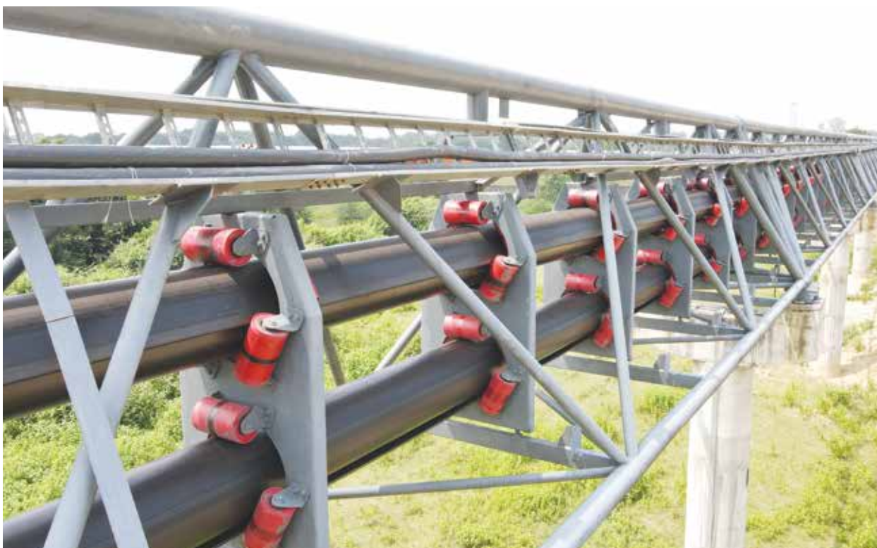
Chandrapur Pipe Conveyor
